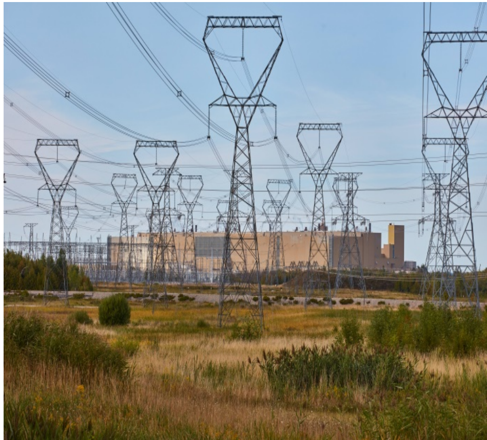
Figure 1: Power Line Infrastructure Connecting Bruce Power to the Electricity Grid
